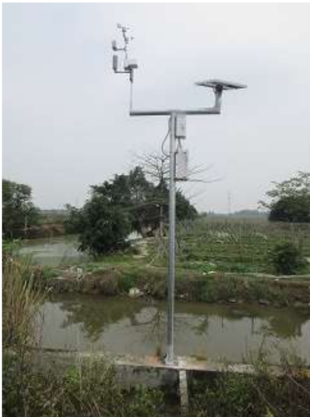
Control box and weather sensor
