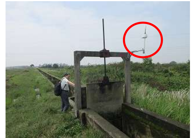
Water level sensor at diversion of An Hoa Canal (An Hoa PS downstream)
